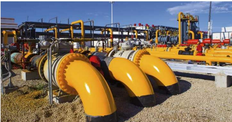
Fig. 96: Typical application field: gas compression station
